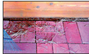
Gap at a fireproof apron
