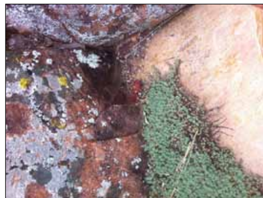
This sedum is coming right out of a crack in the mortar. This is because there's water down behind the rock.
