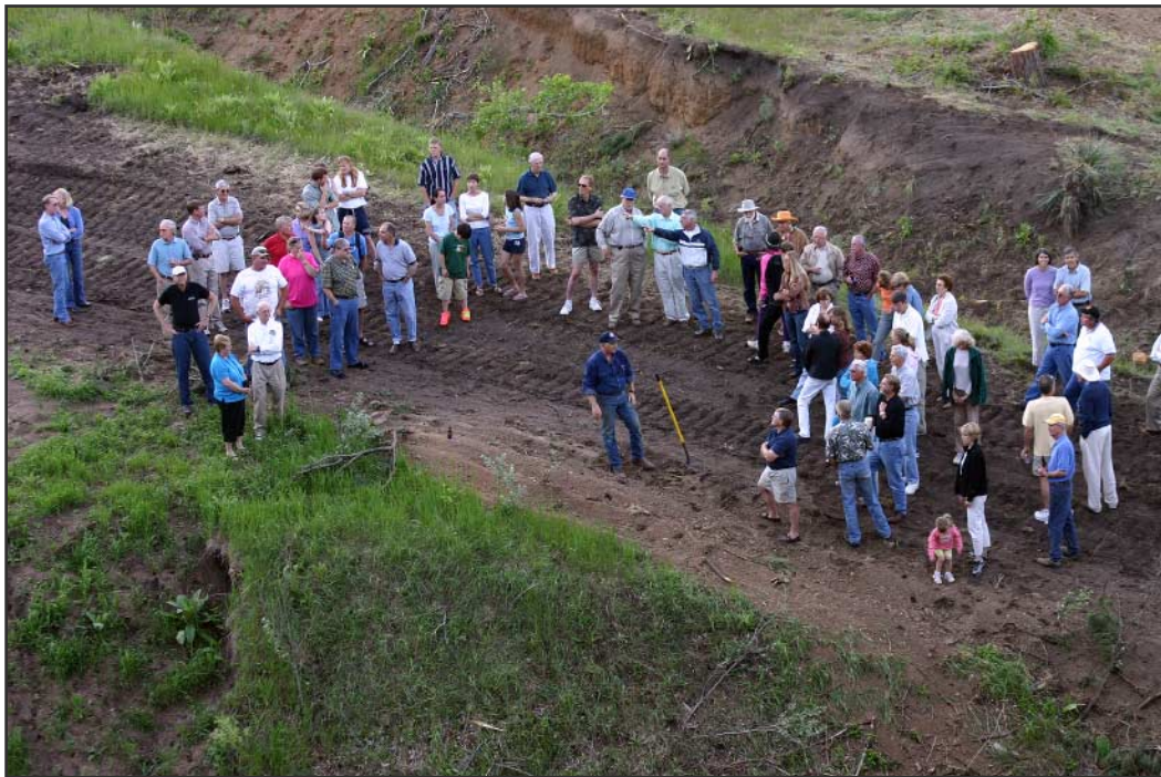
Pine Brookers gather around Water Manager Bob de Haas for the ground-breaking celebration of the new Pine Brook Reservoir.
