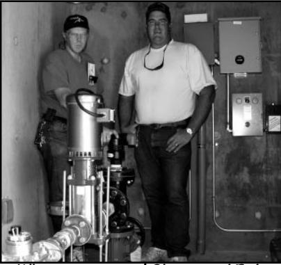
What a contrast! Shawn and Bob deHaas in the new pump house
