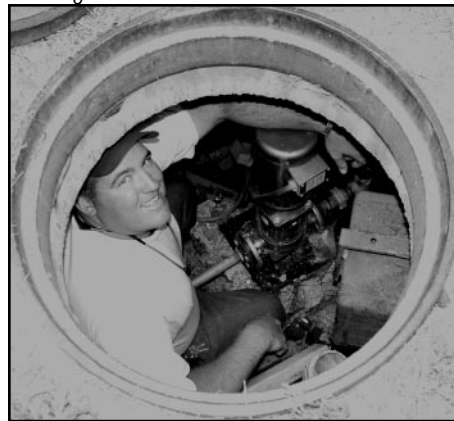
A tight squeeze: Shawn Beauprez tries to work in the old "hole-in-the-ground" pump house at Wild Horse Circle.
