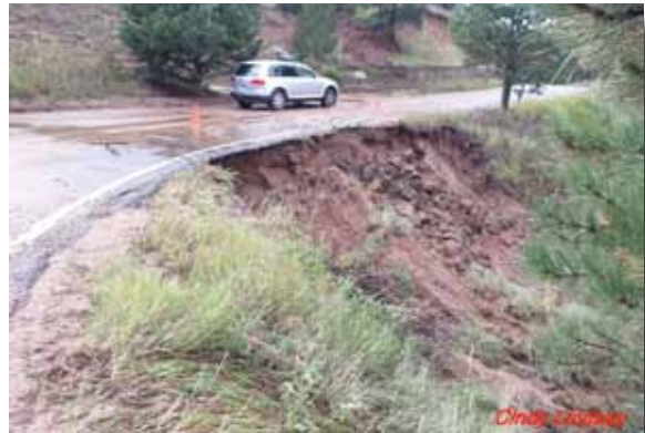
Undercut on Timber Lane.
