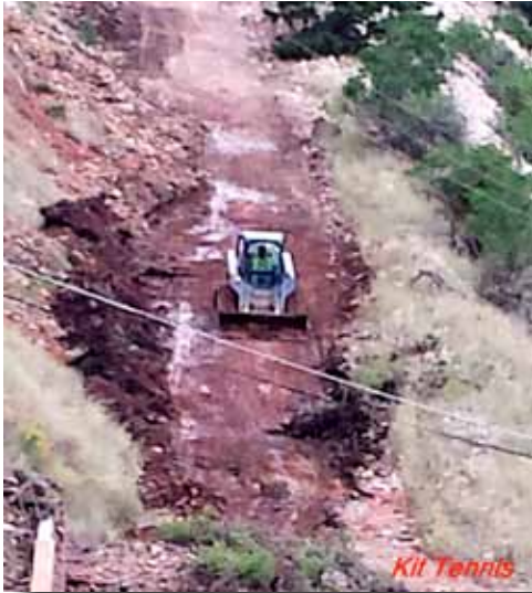
EZ Excavating clearing a path on Fountaintree to access Pine Brook Water Pump house.
