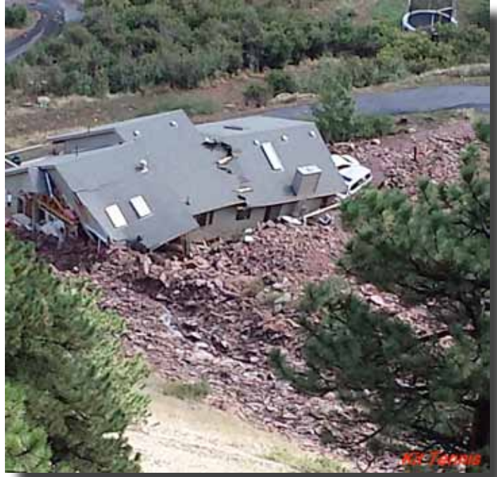
Landslide against the Frisby home on North Cedar Brook.
