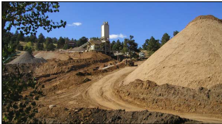
Man-made hills and our own (temporary) cement plant arise near the community center as the reservoir takes shape.
